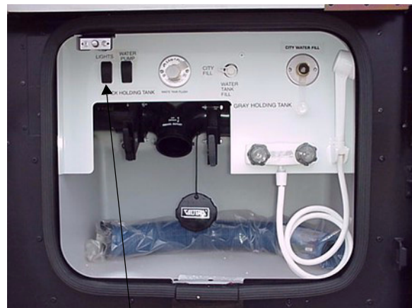
Utility Light Switch
