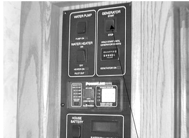
Generator Switch and Hourmeter
