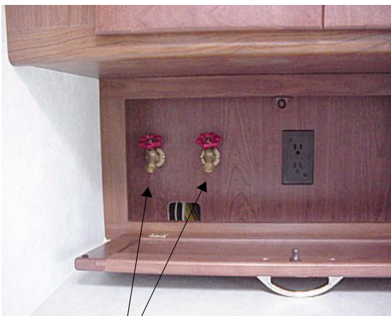
Water Supply Faucets Typical
