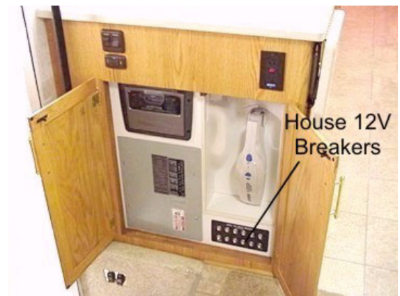
House 12-Volt Circuit Breaker Panel
