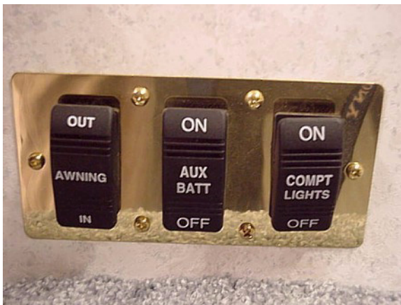
Aux. Batt. Switch (near entrance door)
