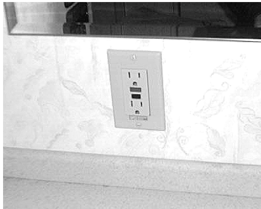
Ground Fault Circuit Interrupter (GFCI)
