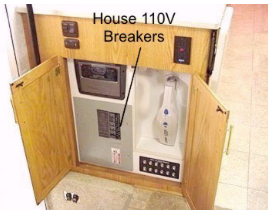
110-Volt House Circuit Breakers
