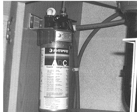
Water Filter Assembly - Below Galley Sink
