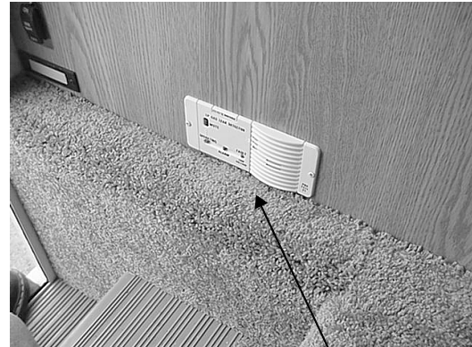
LP Gas Alarm
