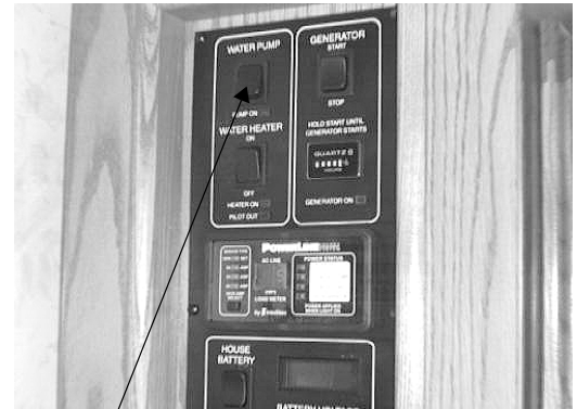
Water Pump Switch
