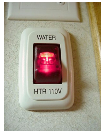
Electric Water Heater Switch (Typical)
