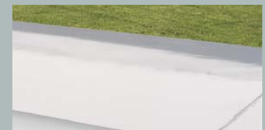
One-year-old Winnebago Industries fiberglass roof
