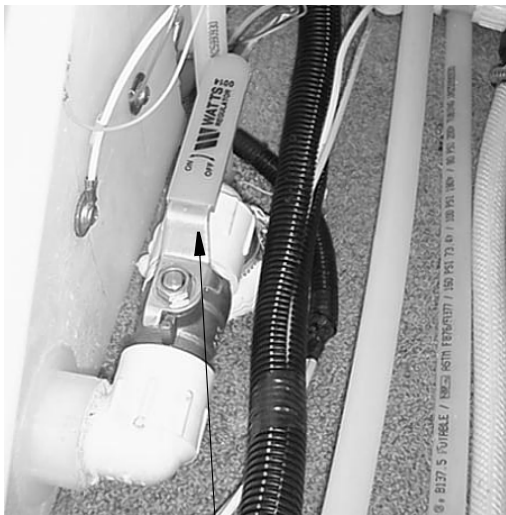
Water Tank Drain Valve (Typical)
