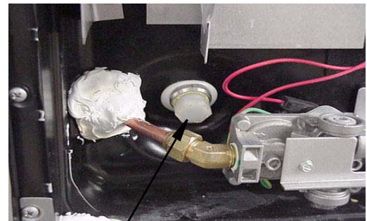
Water Heater Drain Plug Remove with socket
