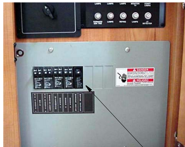
120-Volt House Circuit Breakers
