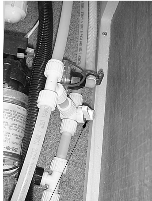
Water Heater Bypass Valve (Typical)
